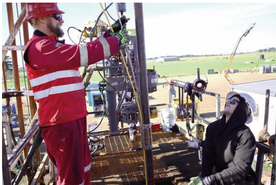
SLB and Wild Desert contractors running cables down the outside of the tubing at CO 2 CRC's Otway International Test Centre Stage 4 injection well CRC-3 (Image: CO 2 CRC)
