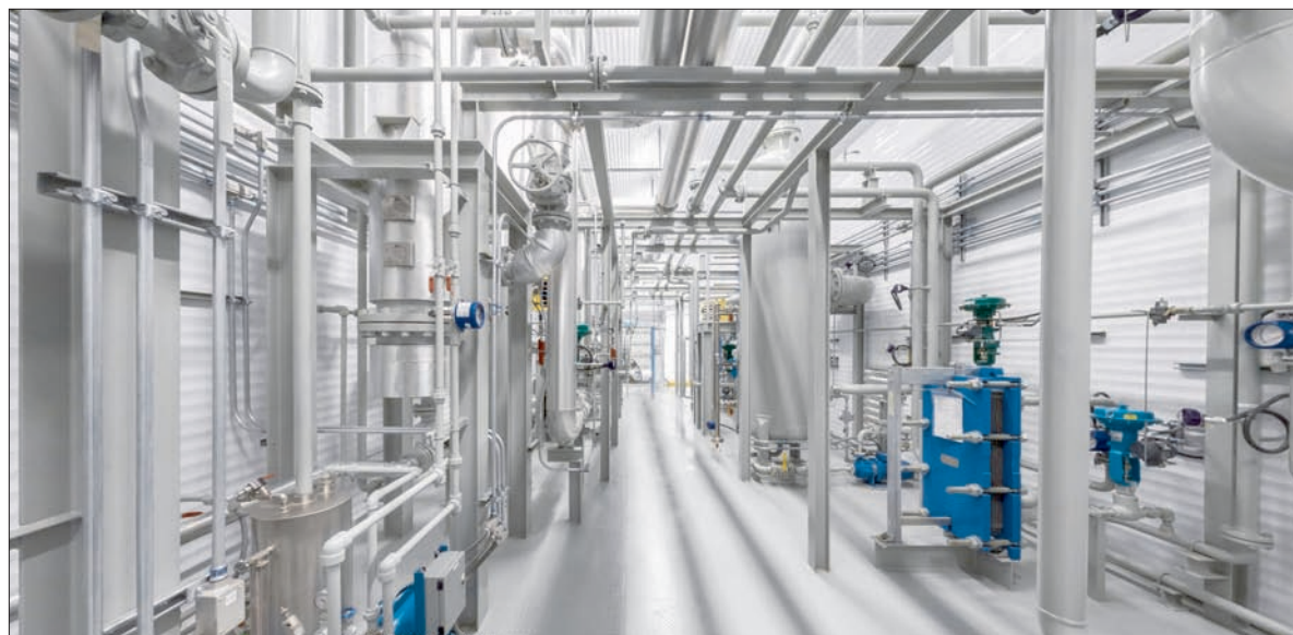
Delta's modularly designed, commercially ready, CO 2 capture unit
