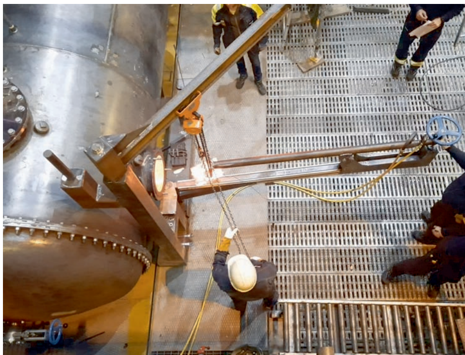
At a pilot facility in Luleå, Sweden, C4U project partners TNO and Swerim demonstrated reheating of steel products with carbon-free hydrogen
